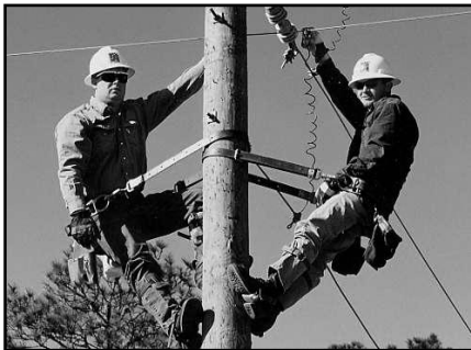
Electric Power Station Repairman Average salary = $65,230/year
